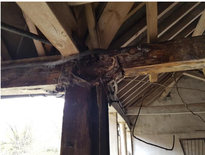
Unit 3 – Decayed Eaves Beam
